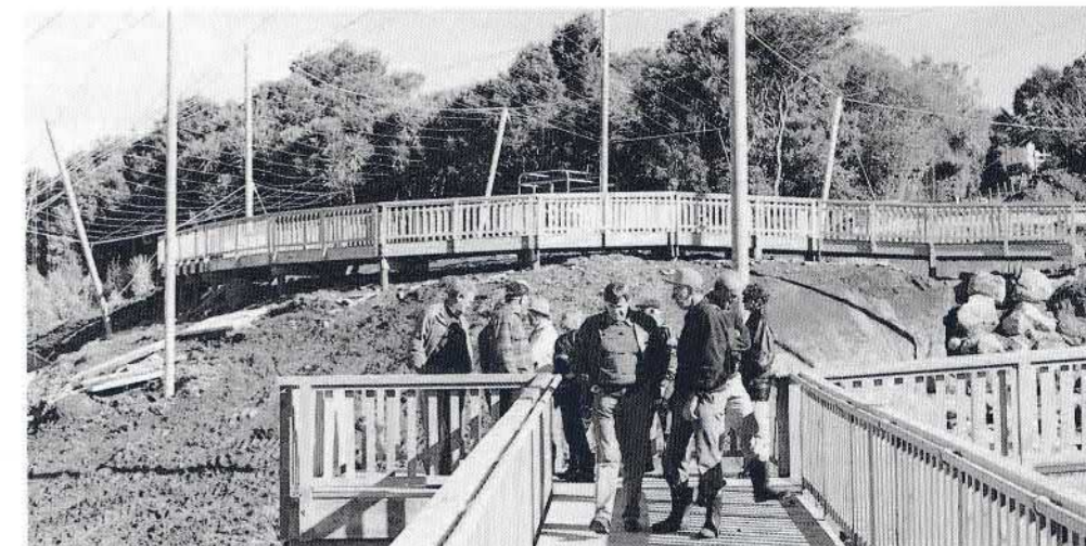
It's hard to appreciate, from a photograph, the sheer size of the new walk-through aviary currently under construction at Hamilton Zoo.
