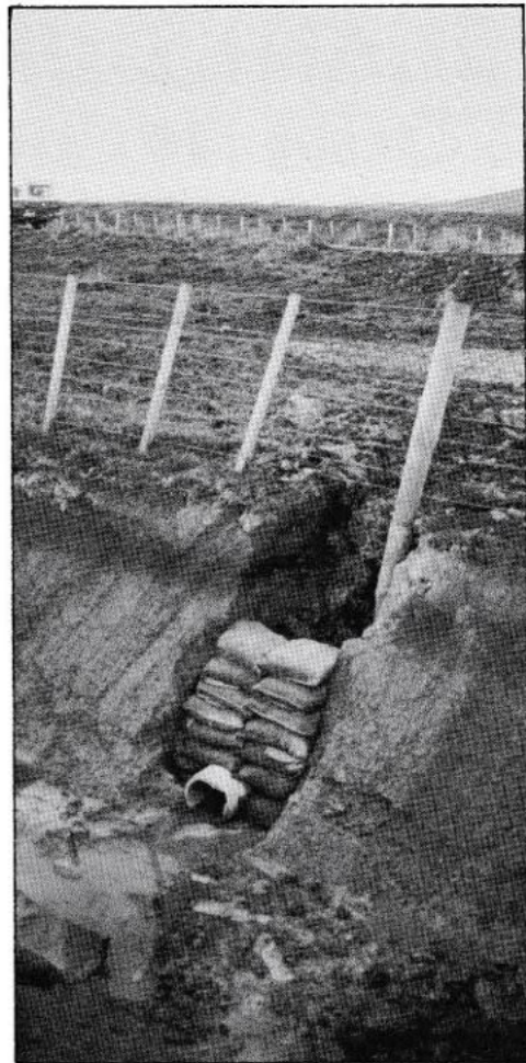
Water begins to flow through the inlet pipe.
