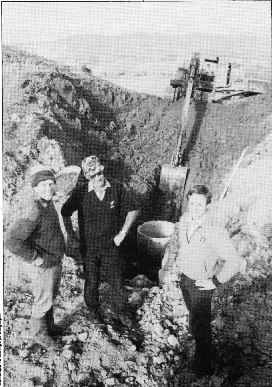
Dennis Handyside, owner of Te Hopai station and Home Lagoon watches excavations with DU President, Jim Campbell and Wildlife Service Officer, Steve McGill. The Ruamahanga River can be seen behind the digger.
