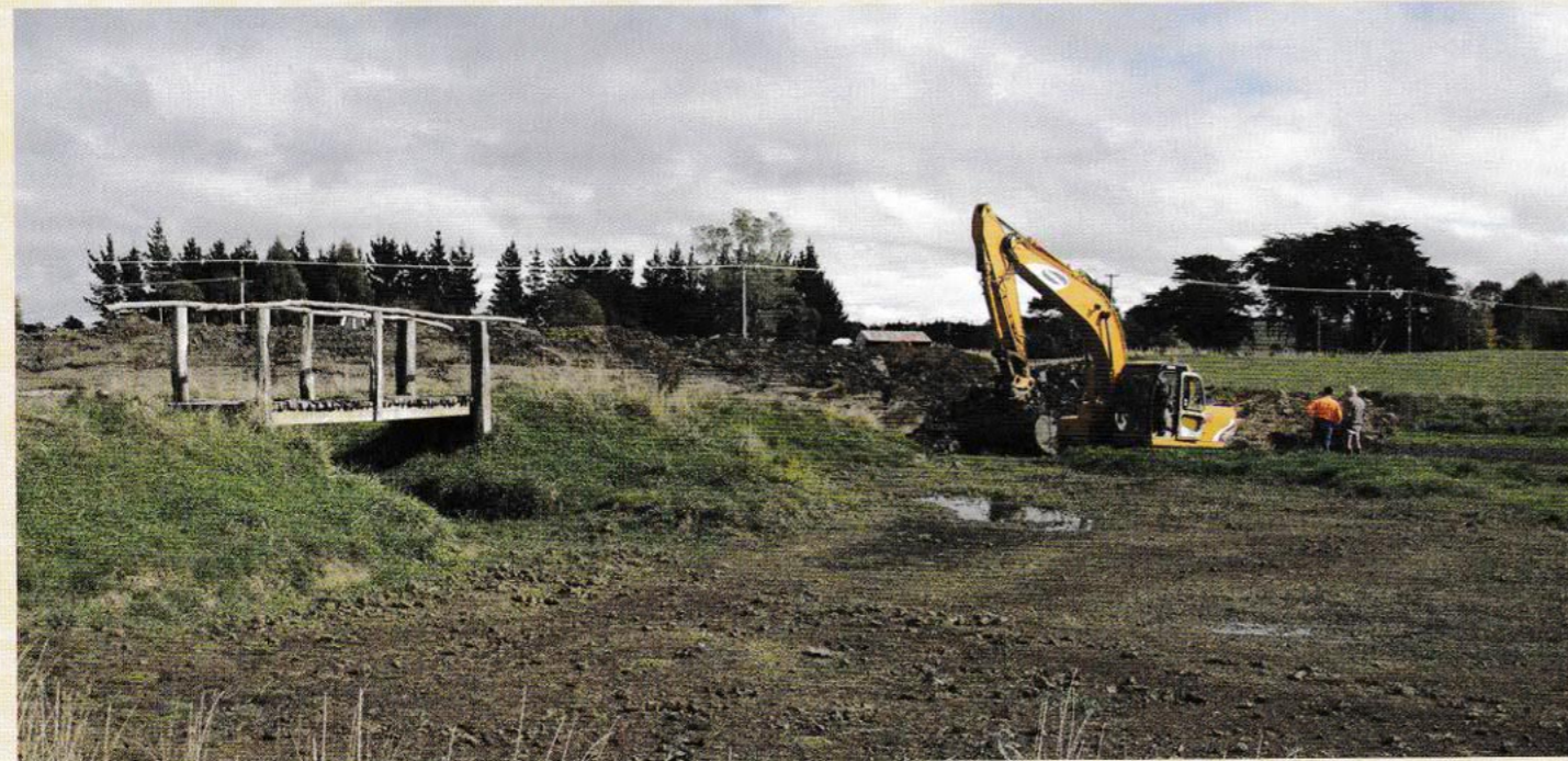
Waterless bridge: The big digger with John Dermer and driver Ray from Tararua Roding enlarging the dam.
