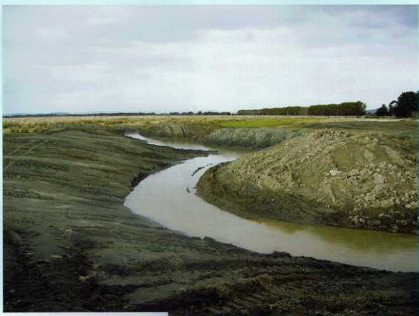
The two photos on right and one below show work on the second stage of developing the Wairio project on Lake Wairarapa. Extensive digging has taken place. Courtesy Ross Cottle
